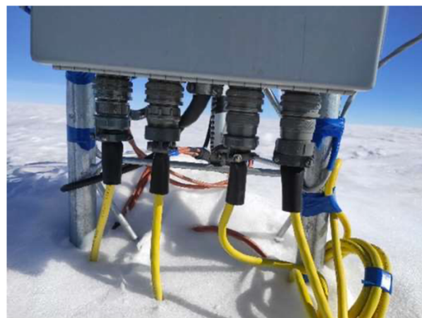
Power switch box. Cables 2 and 3 were loose.
