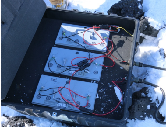
New power system
