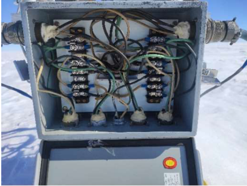
Inside power switch box
