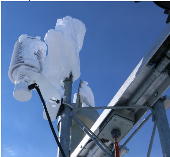
Damage to temperature sensor cable
