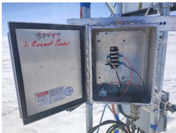
DC2 junction box
