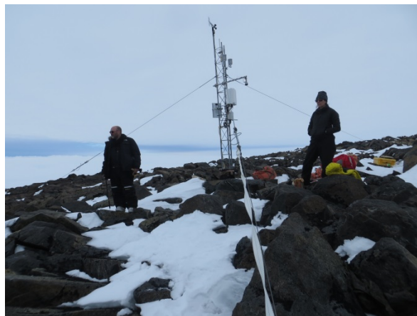
The cargo strap fix on the bad guy wire
