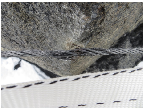
The worn guy wire
