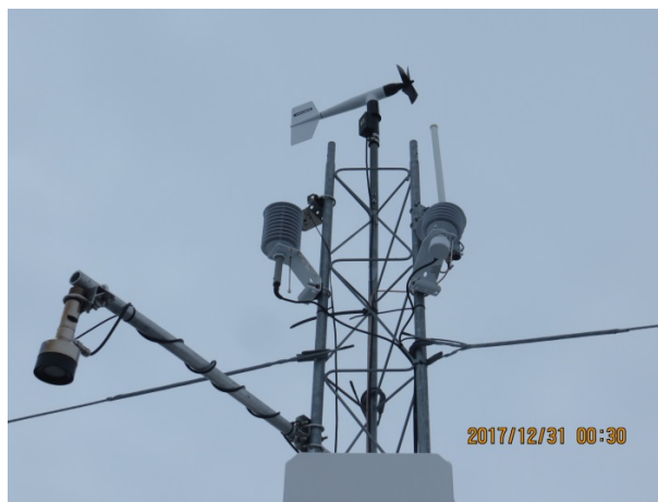
The radiation sensors missing a screw rod
