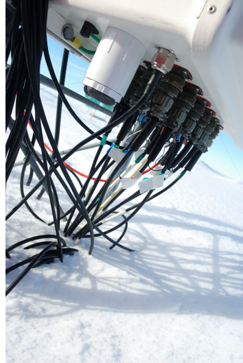
Bottom of enclosure
