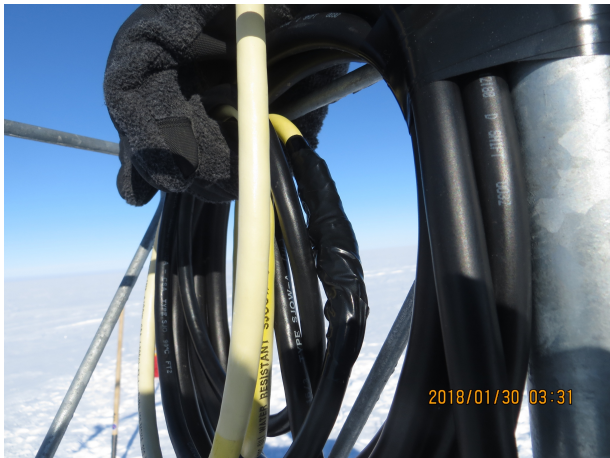
The spliced power cable.
