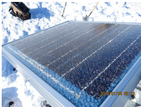
Potential damage to the solar panel
