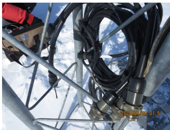
The cable spool. The lower T has white tape.
