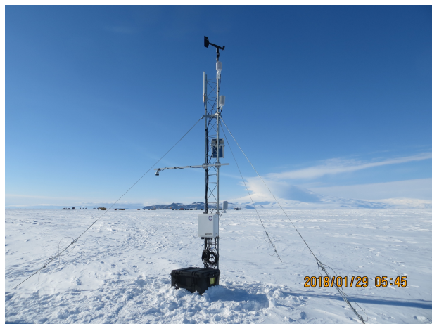
PHX after installing the power system, solar panel, and enclosure.
